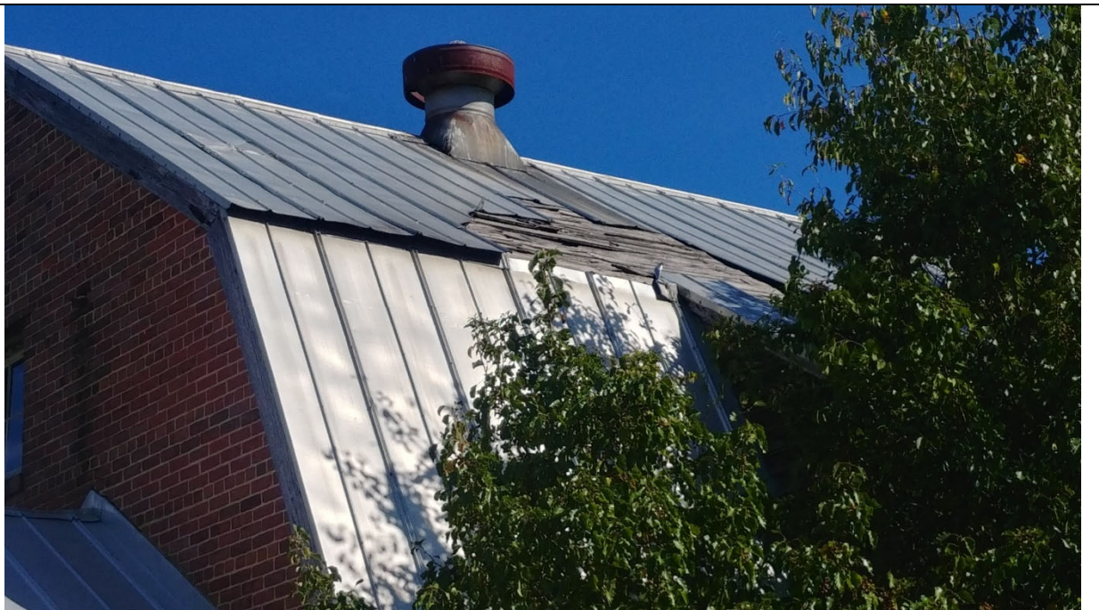
Exterior Roof – Damaged To Be Replaced
