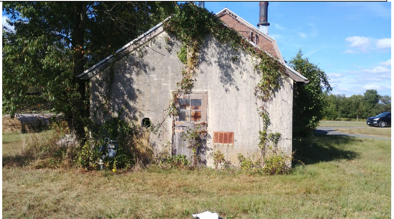
Exterior Masonry Cracks & Structural Damage To Be Repaired
