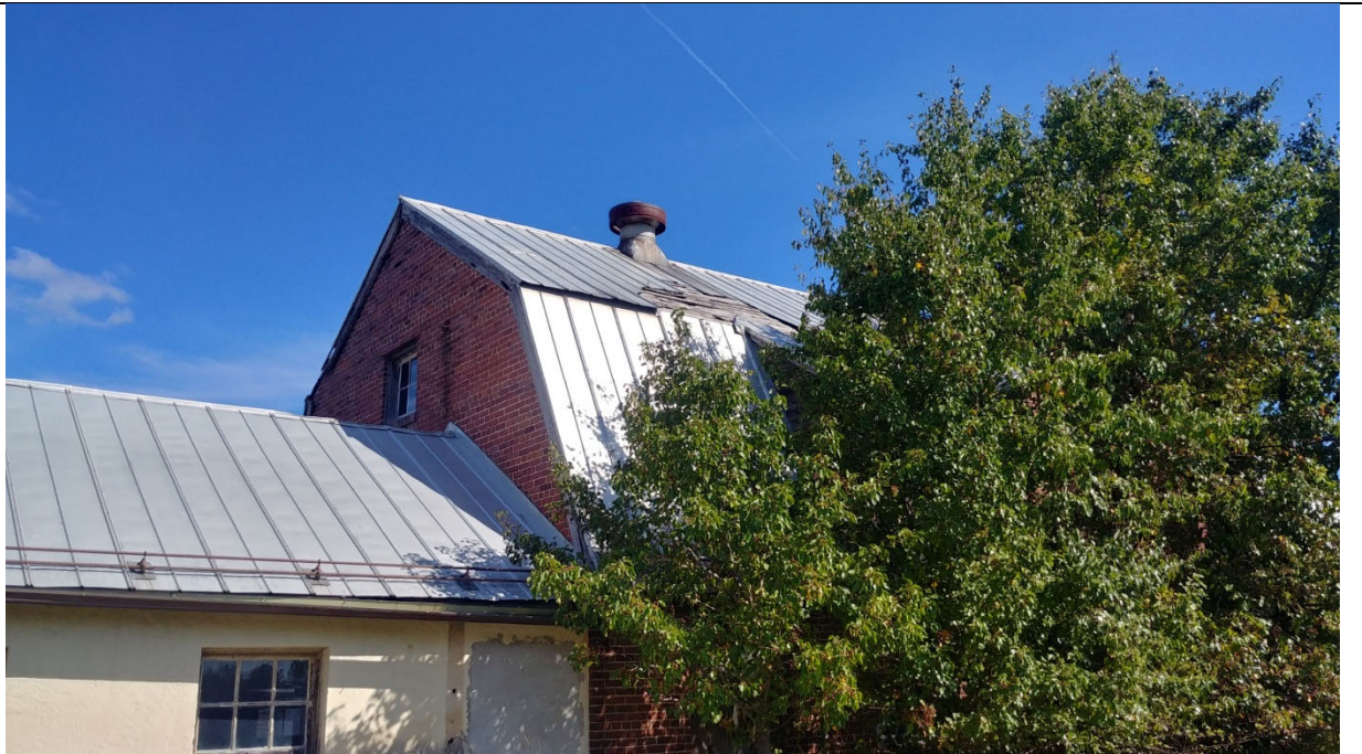
Exterior Roof – Damaged To Be Replaced
